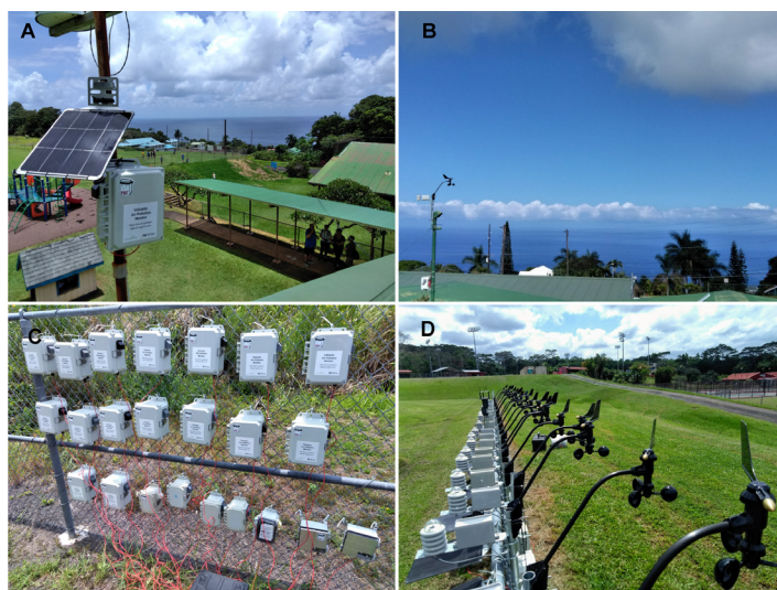
Figure 3. Example a) vog sensor and b) weather station installations on school rooftops. Testing and calibrating multiple c) vog sensors and d) weather stations with reference instruments before deployment at K-12 schools.
